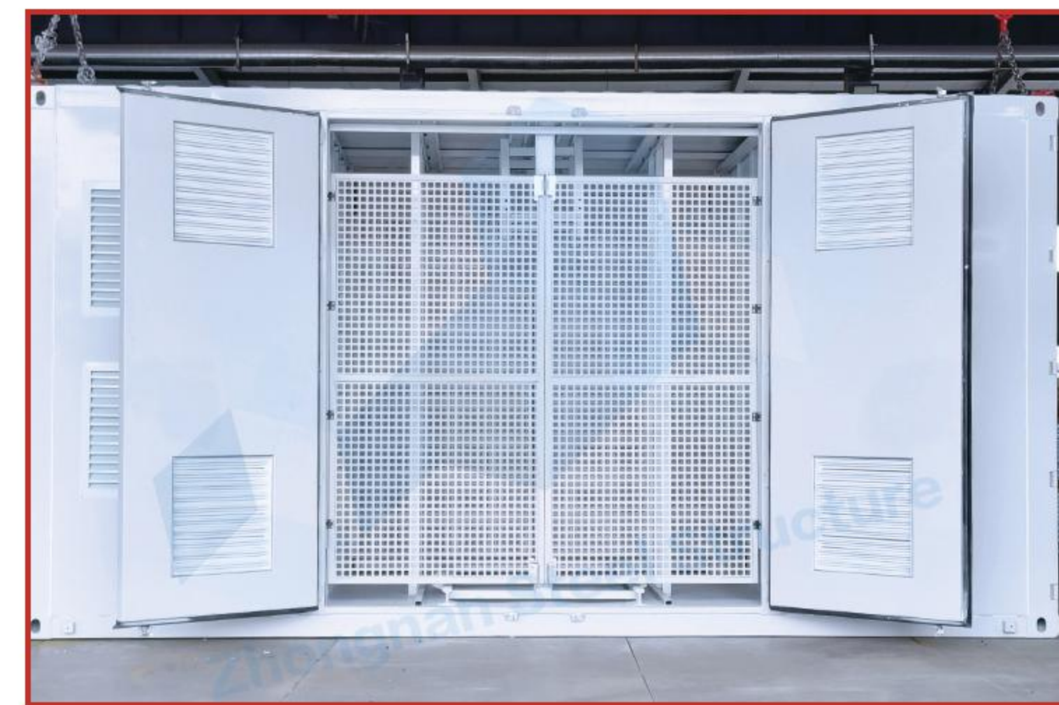
Inside the distribution container
